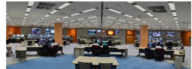
Control room of the Integrated Production Center (IPC)
